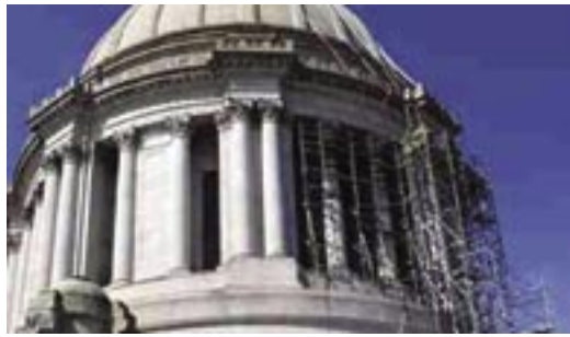
Capitol front with exterior scaffold, not chosen as route for shotcrete hose
